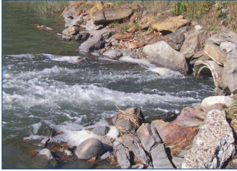
Upstream end of perched culvert under Long Reach Lane, while tide is dropping
