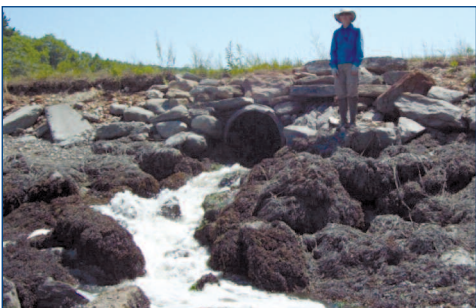
Downstream end of perched culvert under Long Reach Lane, while tide is dropping
